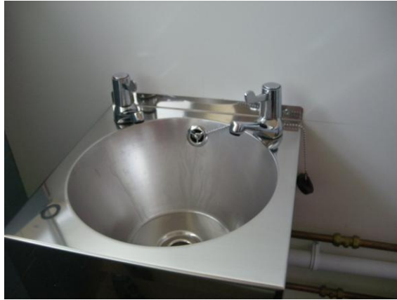
Picture 5 Inappropriate hand washing sink
