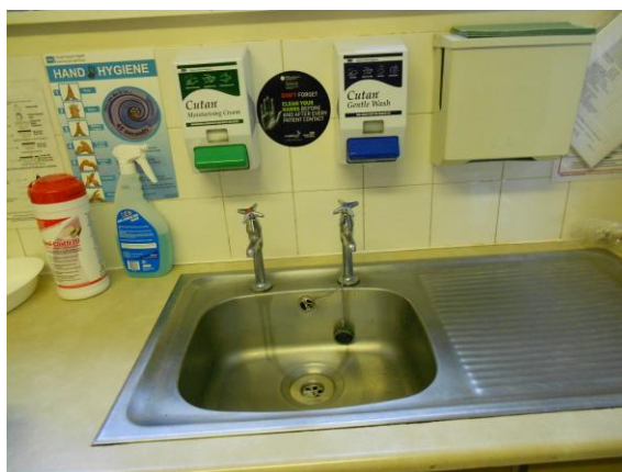
Picture 5 Treatment room sink, twist taps, overflow and plug insitu
