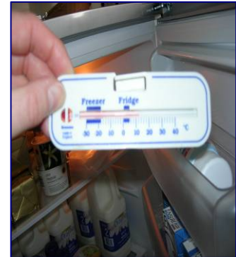
Refrigerator not achieving required temperature
