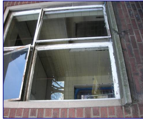
Window frames poor state of repair
