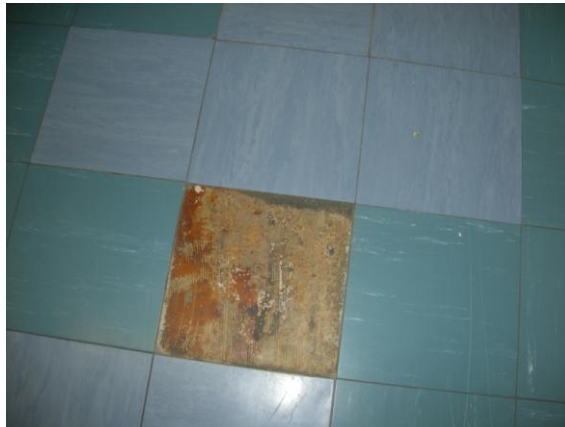
Picture 3 Ward 4 South damaged flooring
