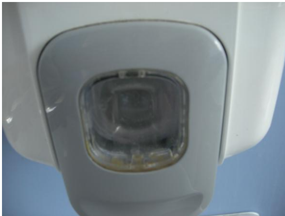
Picture 5 Ward 4 South dirty soap dispenser
