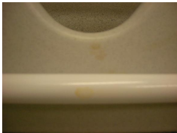
Picture3 Stained underside of commode
