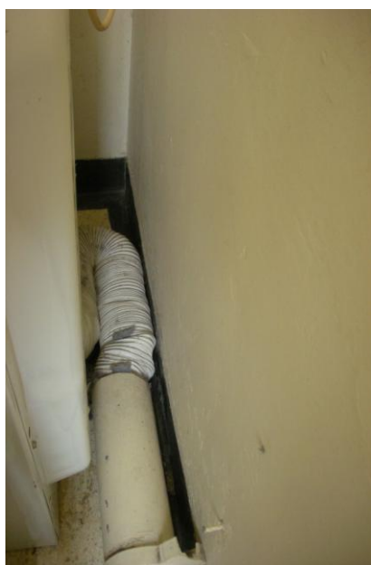
Picture 4: Poorly fitted tumble dryer vent, dust and balls of lint
