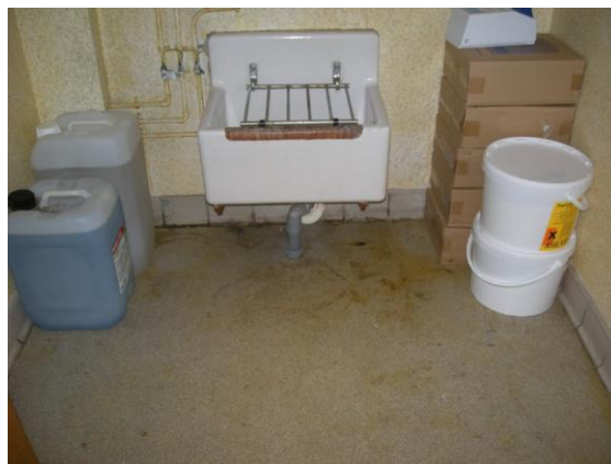
Picture 3 - Ground in stains on domestic store floor
