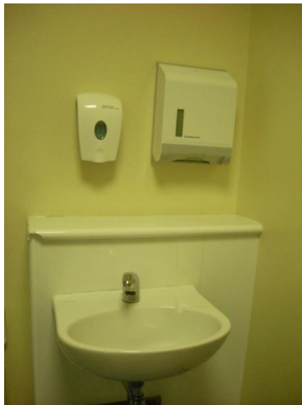
Picture 6 New hand wash sink with soap and hand towels available
