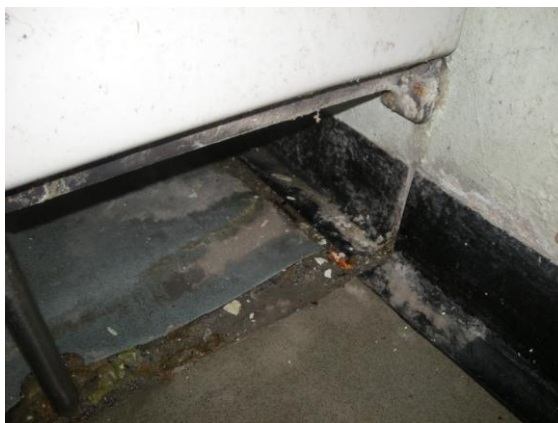
Picture 4: Damaged flooring and wall
