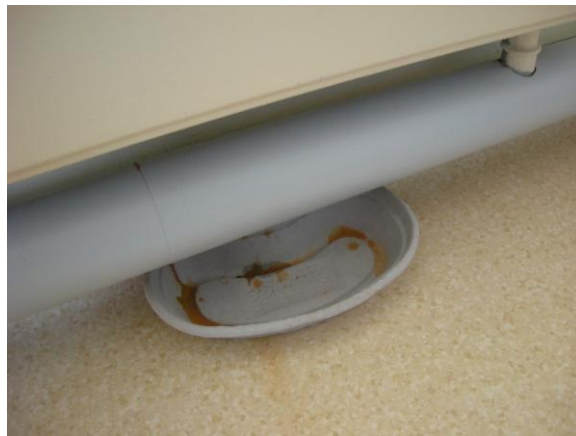
Picture 2 Exposed leaking pipe
