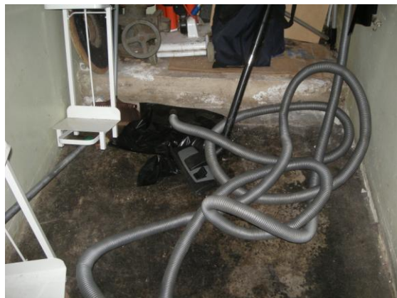
Picture 4 Cleaning store with unfinished floor
