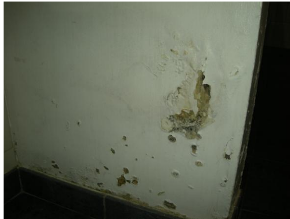
Picture 3 Damage to wall in public toilet
