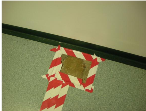
Picture 2 Damaged Floor
