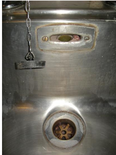
Picture 4 Hand wash Sink in Clean utility room
