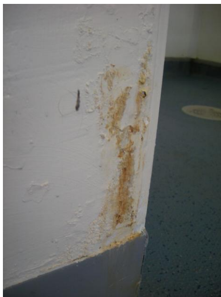
Picture 2 Shower wall damaged, discoloured and flaky paint
