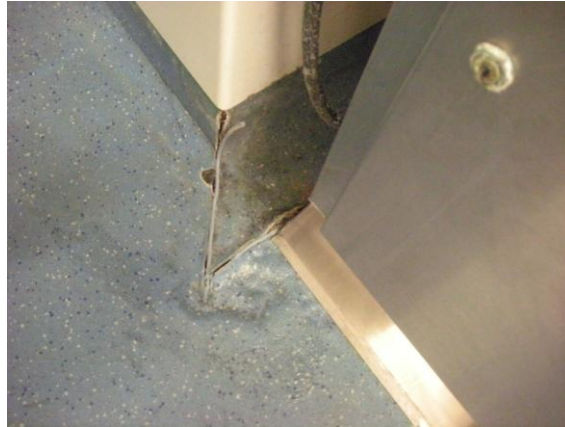
Picture 1 Damaged flooring
