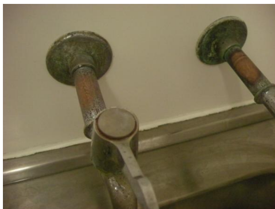
Picture 2 Corroded taps
