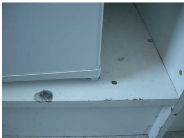
Picture 2 Clinical room - dusty, damaged shelving
