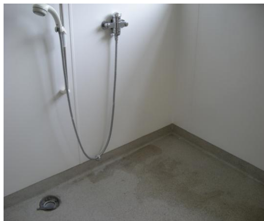
Picture 3 Missing shower outlet
