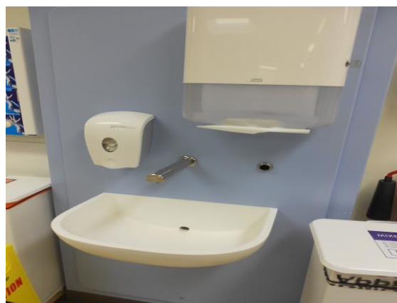
Picture 2: Newly installed hand washing facilities
