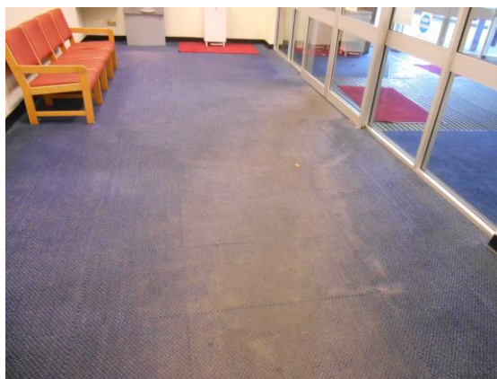
Picture 2: Worn carpet at Hospital entrance
