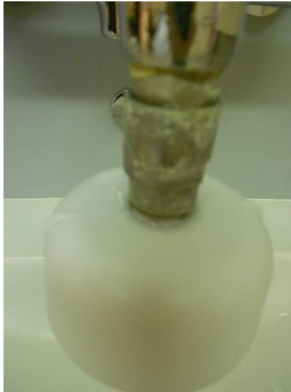
Picture 5: Limescale on tap
